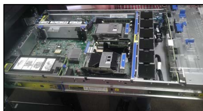
Server Builds & Remote Login Access
